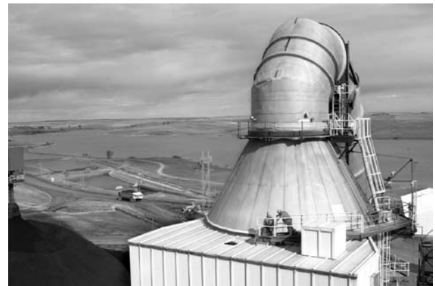
As part of the Minnkota settlement agreement, the Young 2 sulfur dioxide scrubber will be modified in 2010 to increase its removal efficiency. A new scrubber will be constructed for Young 1 in 2011.
